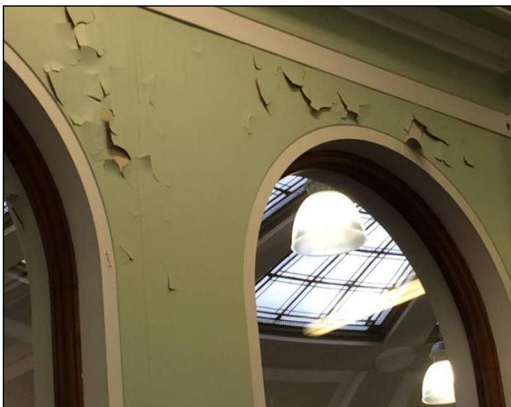
3 - Paint peeling from walls and ceiling
